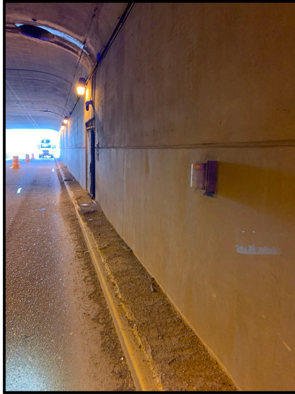
Fire Alarm Station
